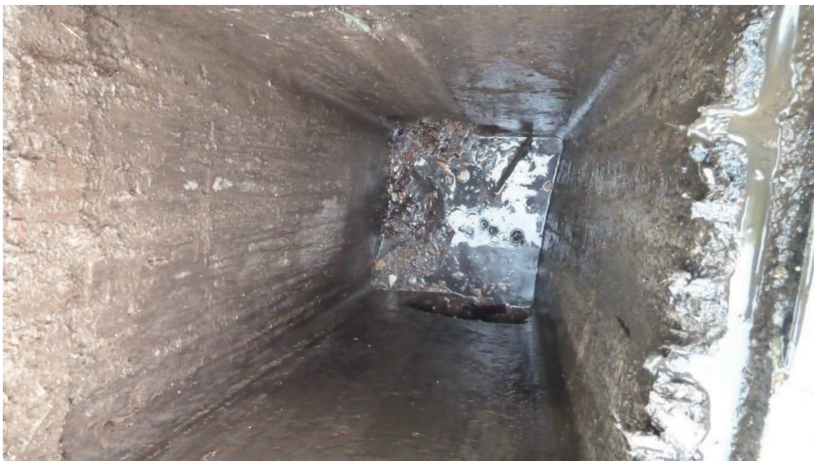
Figure 18. Avaloir A4 bassin versant C - A nettoyer
