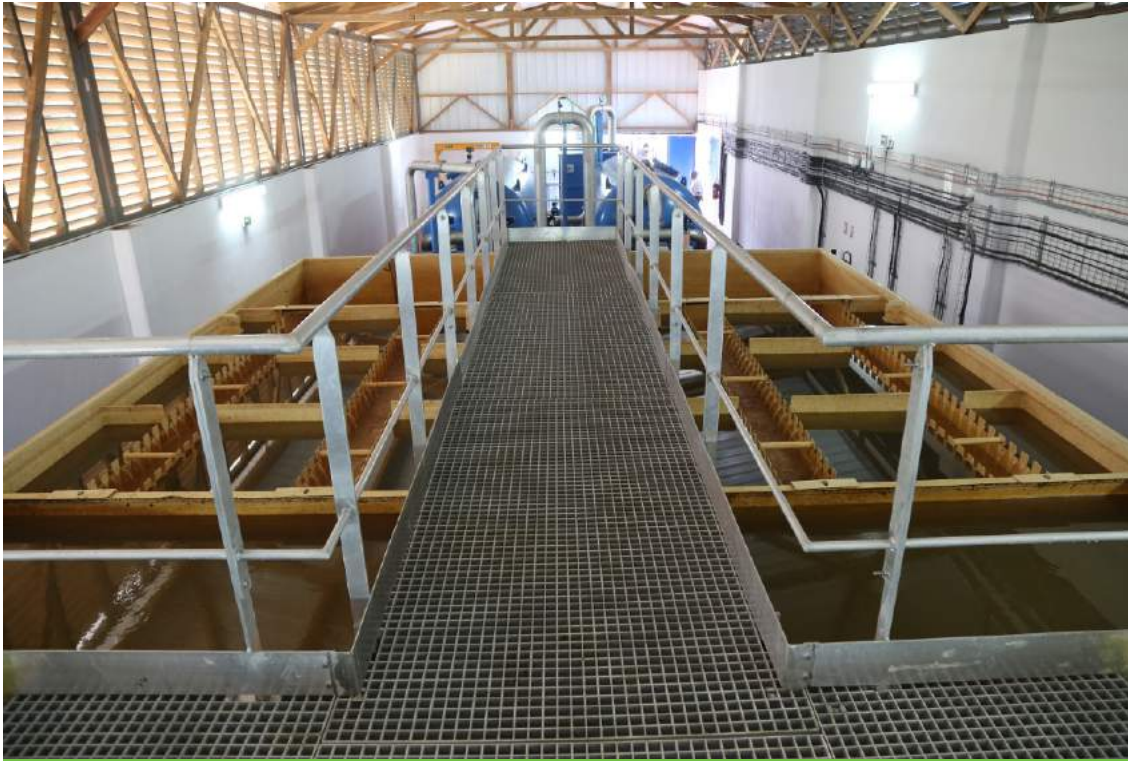
Station Eau Potable - Saint-Laurent du Maroni
