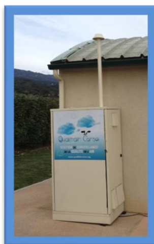
Figure 7 : Station mobile : l'armoire mobile
