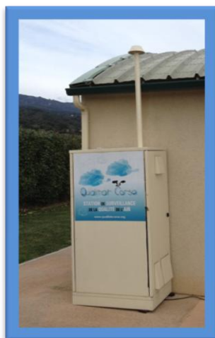
Figure 7 : Station mobile : l'armoire mobile
