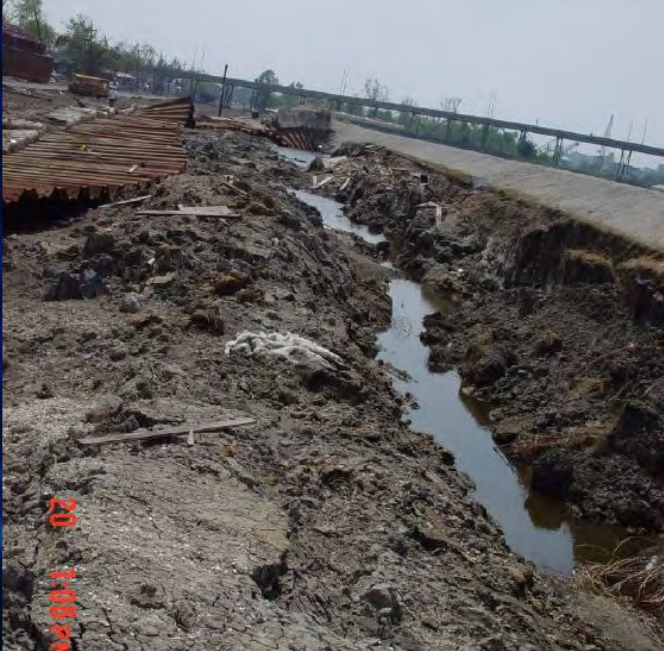
Figure 11-5. Scour and Erosion Leading to the Failure of the I-Wall on the IHNC Adjacent the South Breach (9th Ward)
