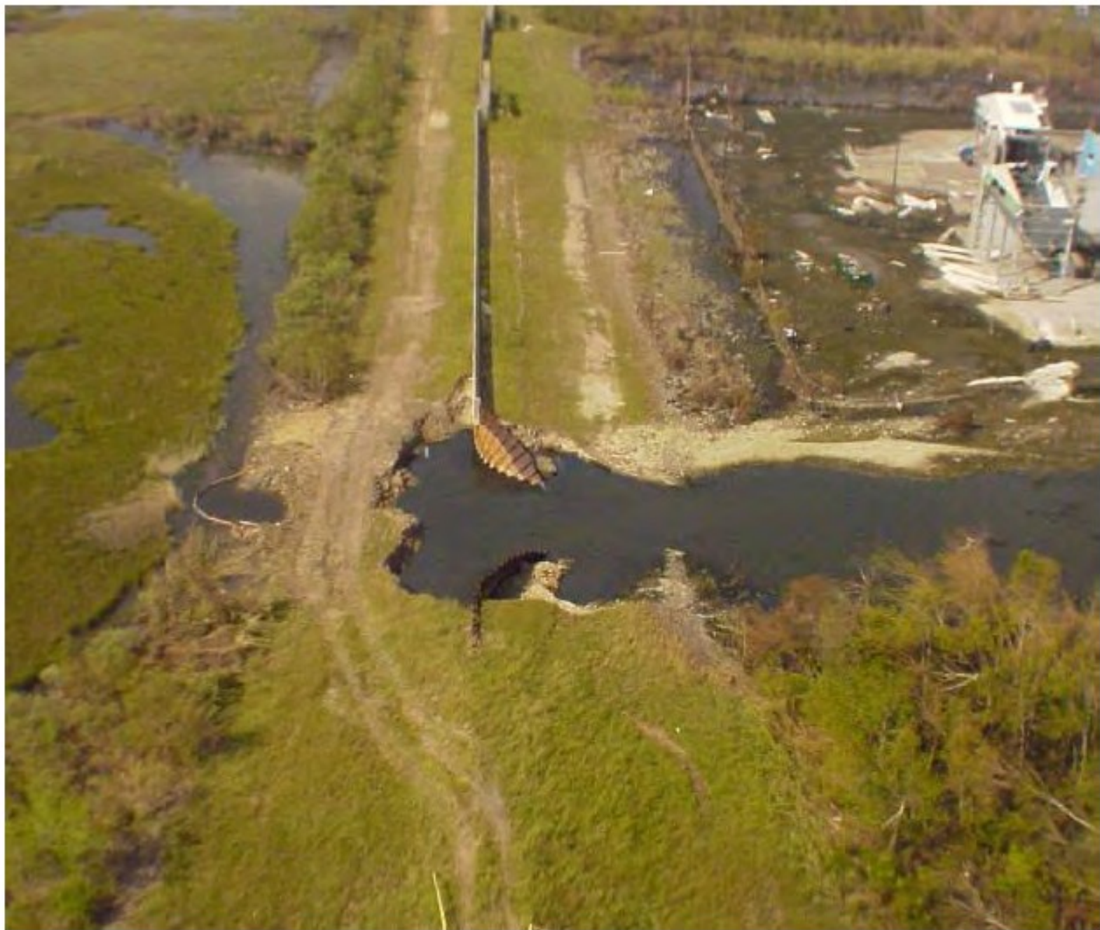
Figure 12-44. NOE3_D Sheetpile Wall Failure (near Sta 772+00 B/L New Orleans East Back Levee) (Coordinates 30 deg 01 min 04.30 sec N, 89 deg 53 min 49.36 sec W)
