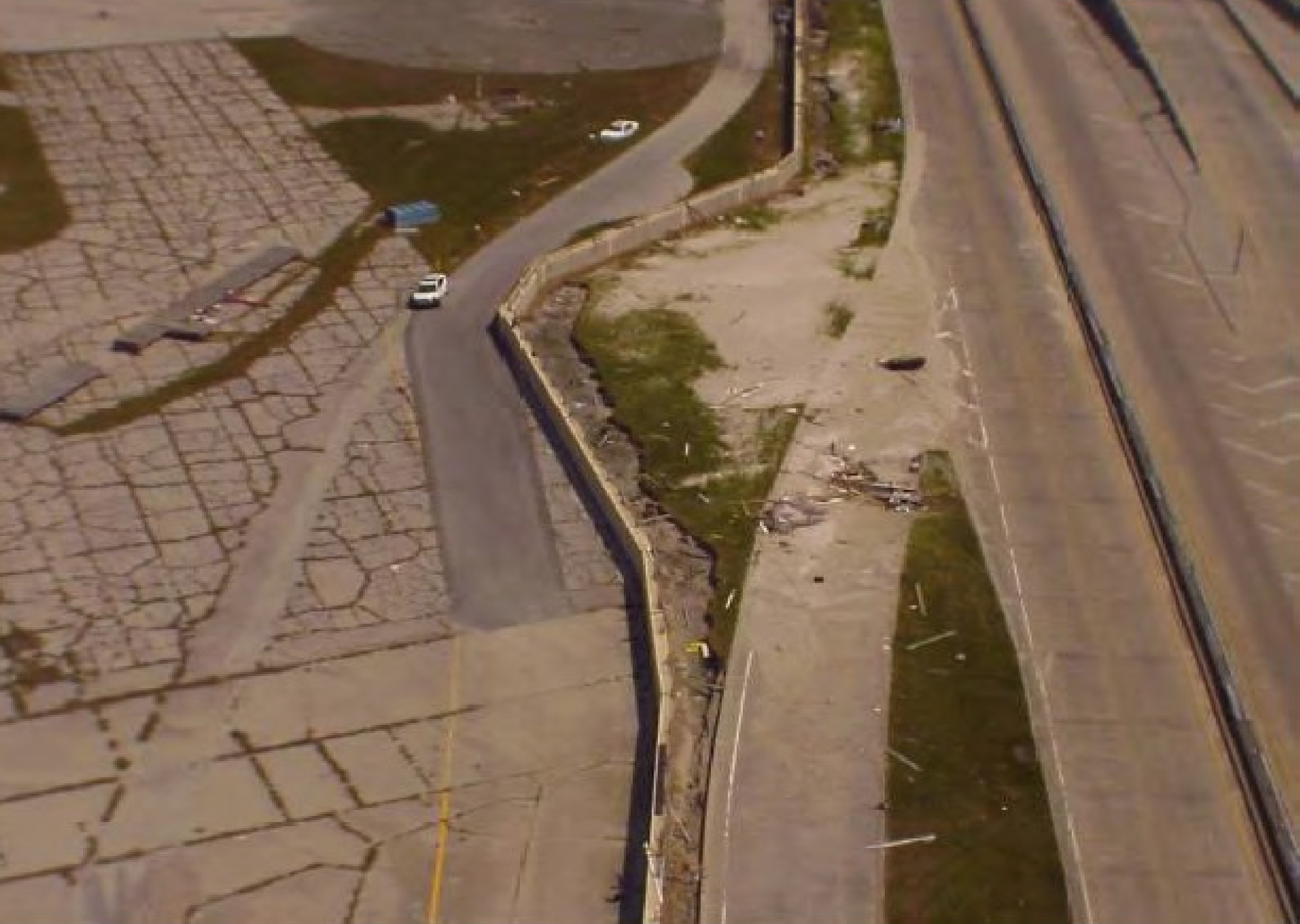
Figure 12-6. NOE6_B. Scoured Section on Protected Side at Lakefront Airport Floodwall
