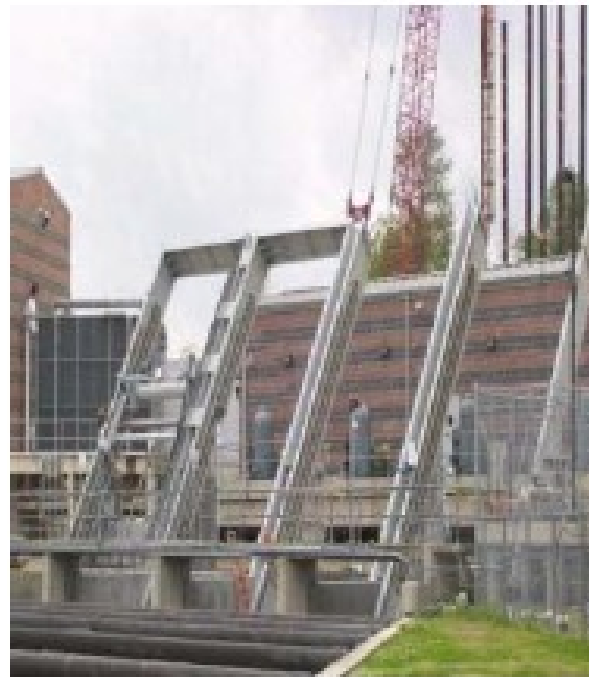
Storm proof 49 pump stations ($322 Mil)
