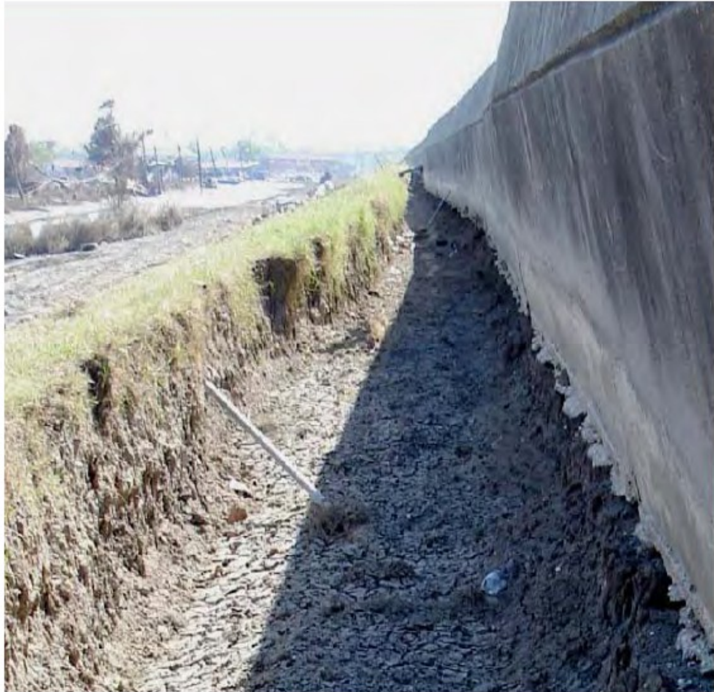
Figure 11-4. Scour and Erosion on the Protected Side of the IHNC Adjacent to the Ninth Ward in the Vicinity of the South Breach
