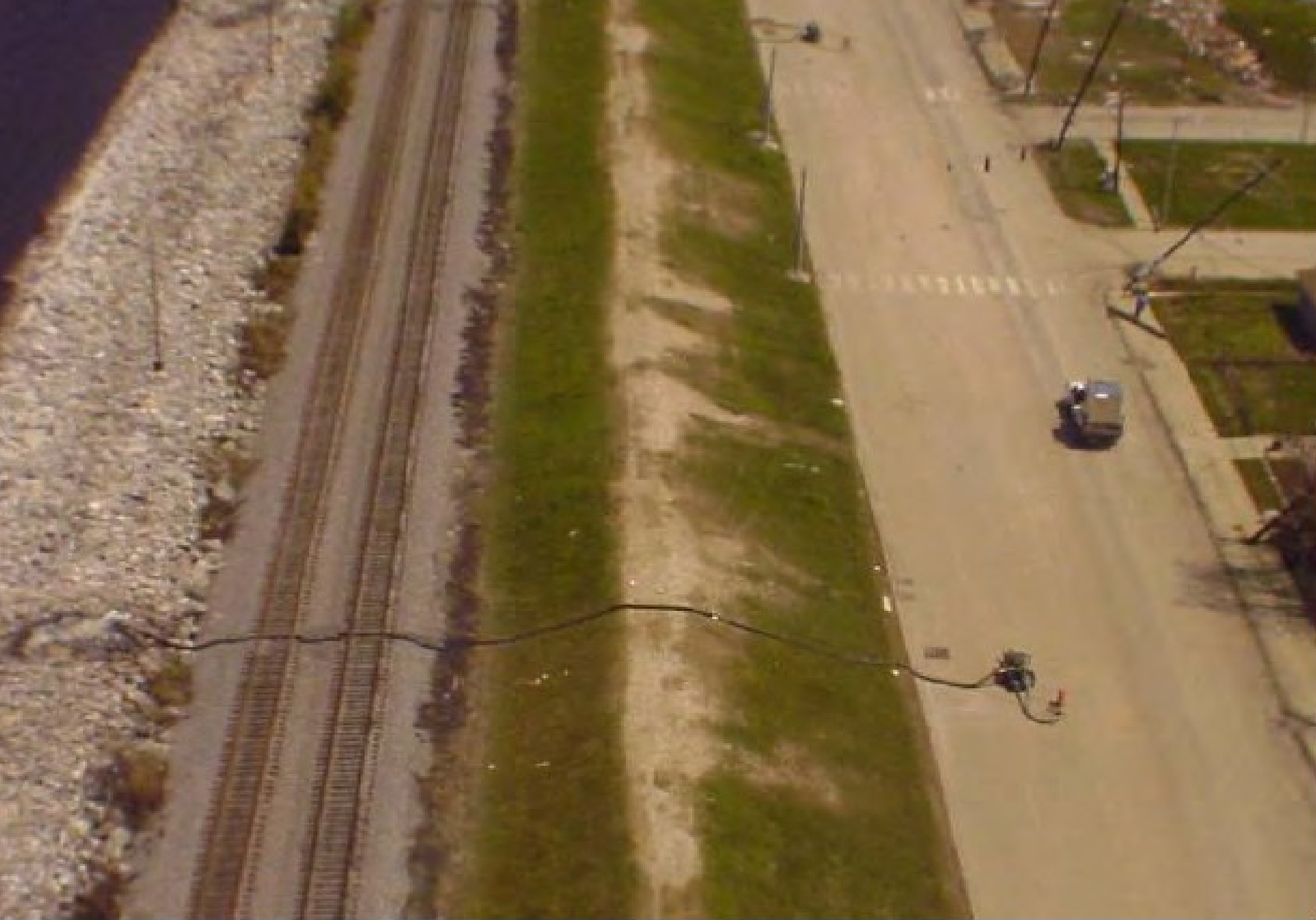
Figure 12-10. NOE7_B Typical Crown and Landside Scouring
